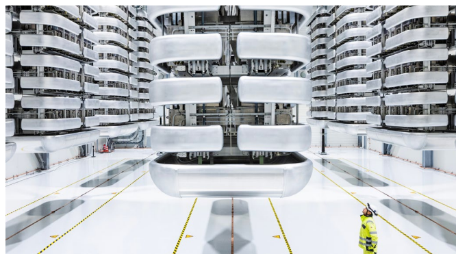
Picture: inside a converter station, photo credit: Hitachi Energy
