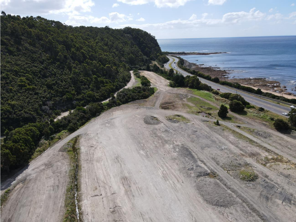
Photo 5-2 Heybridge Converter Station site (where HDD launch pad site would be located), looking north-west
