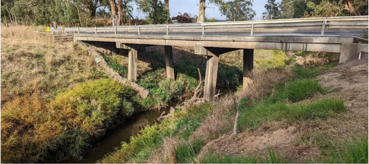
Figure 86. Looking downstream at the Tarwin River East Branch bridge crossing on Meeniyah-Mirboo North Road with flood debris in channel and on left bank
